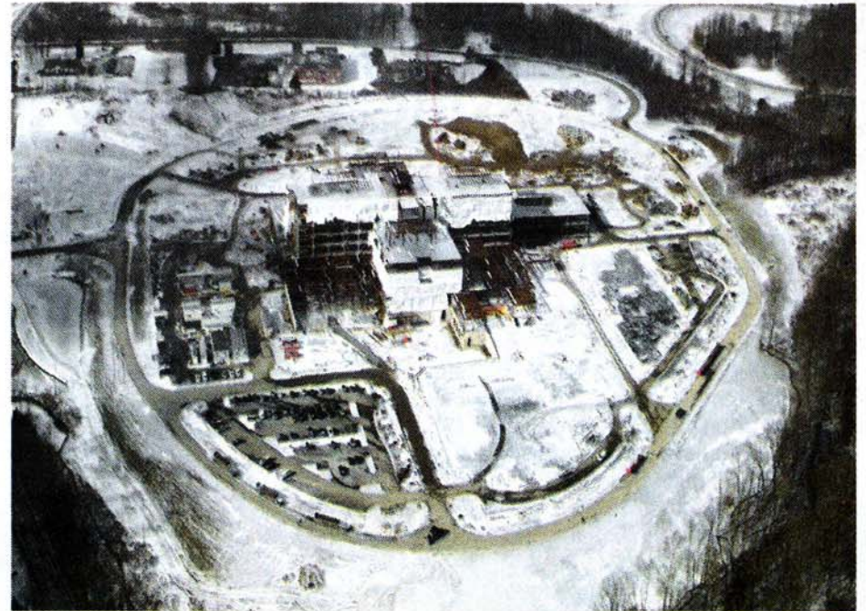
The new hospital for Orange Regional Medical Center recently celebrated a 'topping out.'
